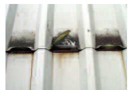
Leathergrain alternative on hot dip galvanized steel substrate roof after 7 years.
